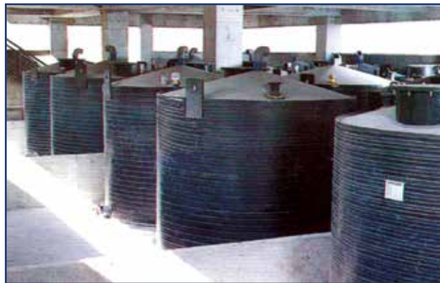
Picture 5.1 - Dizayn PE tanks being used for chemical storage.
